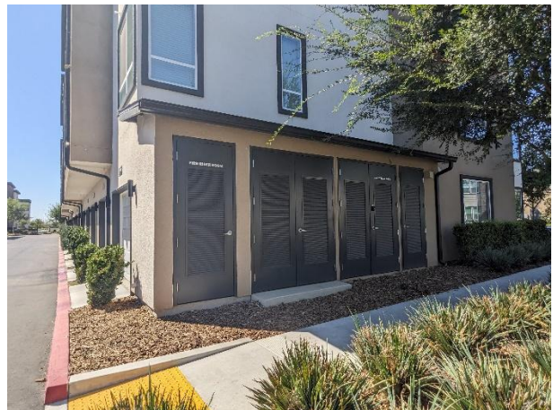
Example of utility enclosure.
